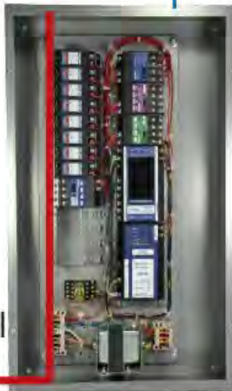
Master Relay Panel
